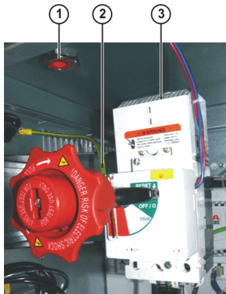
Fig. 4-5: Power supply connection at main switch
