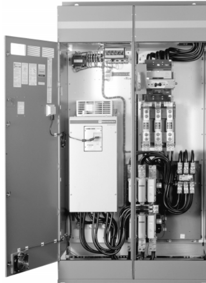
MCC ALTISTART Unit with Open Door
